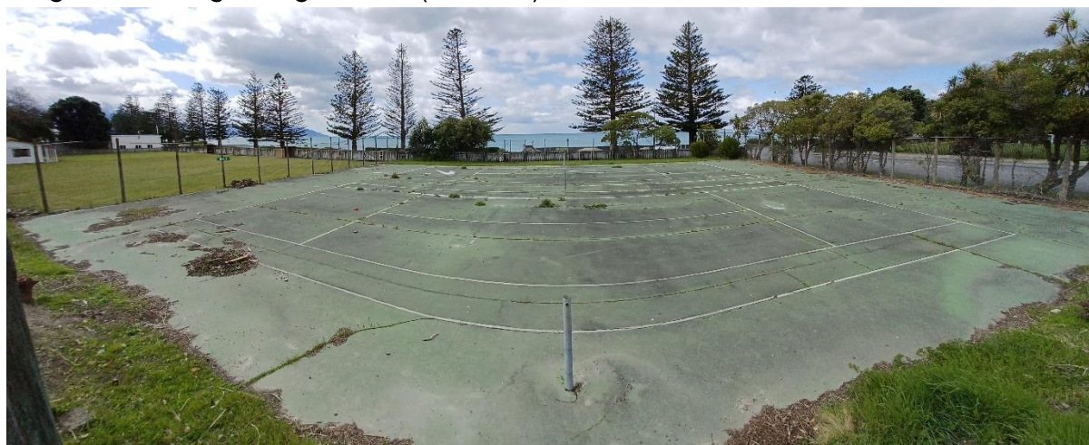
Image one: Existing damaged courts (lower tier)
